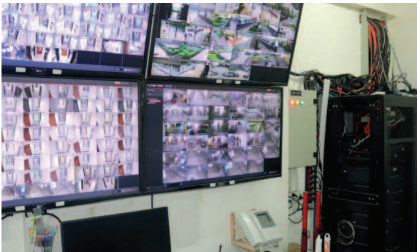
TRẠM KIỂM SOÁT TRUNG TÂM ( Central Control Station )
